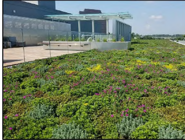
EXTENSIVE GREEN ROOF PLANTED WITH SEDUM MAT
