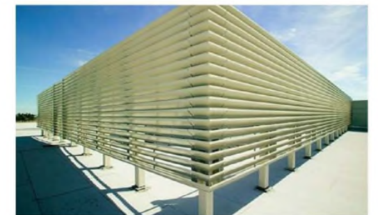
5. PENTHOUSE EQUIPMENT - SCREEN
